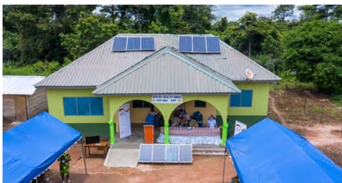
Picture 2: Commissioning of Solar PV at a Rural Clinic
